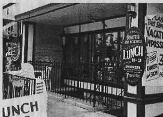
The storefront of this building has been completely removed. The setback of the new storefront is out of alignment. To preserve the historic setback, do not remove the front wall or storefront.
